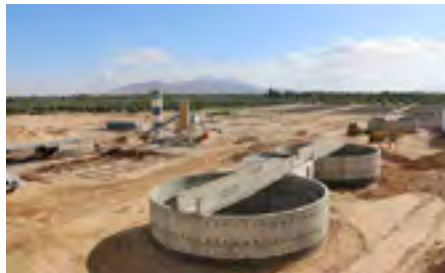
STEP de GAFSA (Tunisie) Water treatment plant of Gafsa (Tunisia)
