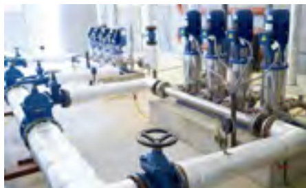
Station de pompage de TASSETTE (Sénégal) Water pumping plant of TASSETTE (Senegal)
