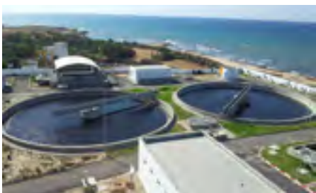
STEP de NABEUL SE4 (Tunisie) Water treatment plant of Nabeul SE4 (Tunisia)
